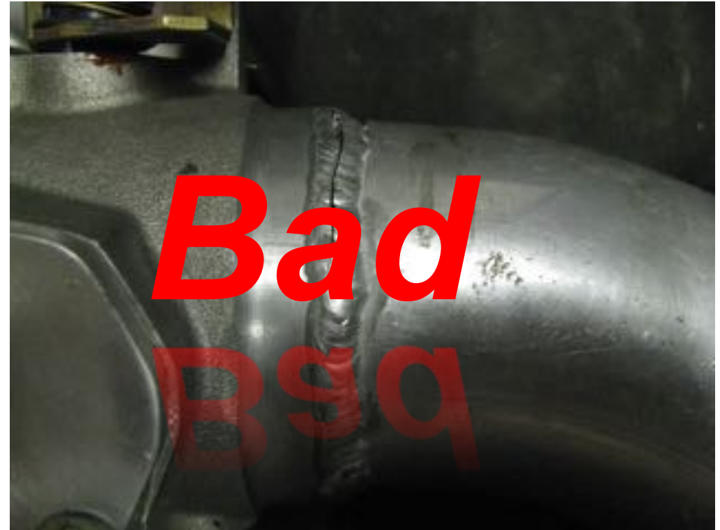
Cracked welded pipe knee joint
